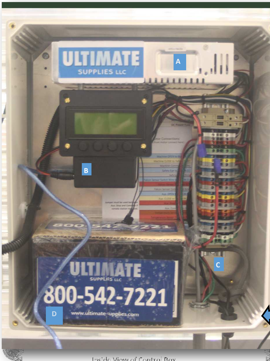
Inside View of Control Box
